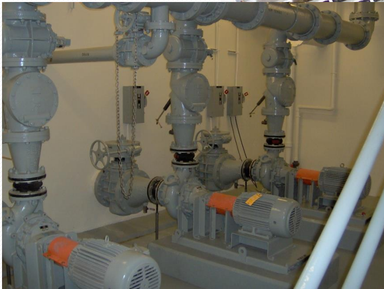
Raw Sewage Pumps
