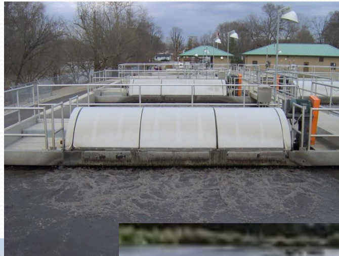
Vertical Loop Reactor
