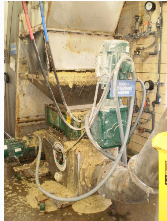
Excessive Grease in Bar Screen
