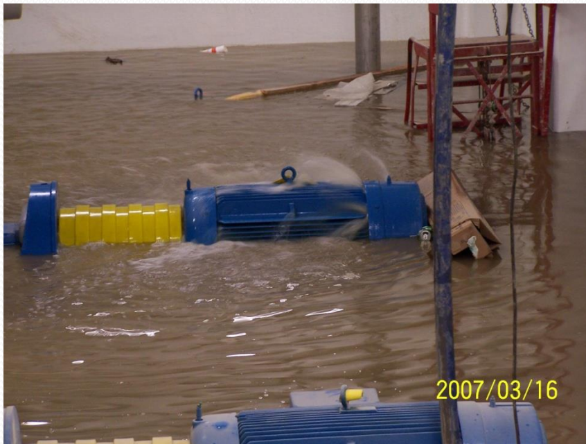
Dry Pit Pump Basement
