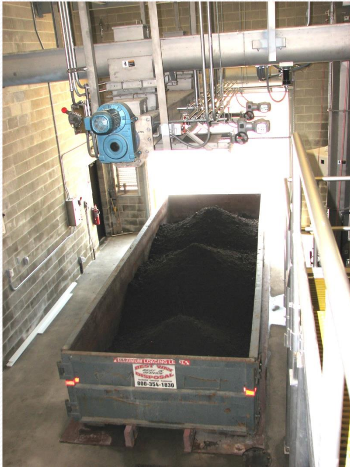
Dewatered Sludge from Belt Presses to Landfill
